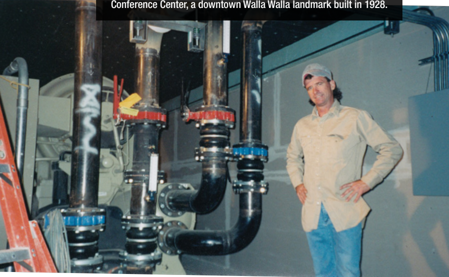
Local 598 members Jeff Goldsbury (top) and Ray Kreuger (bottom) inspect the hydronic heating and cooling system installed during the 2001 complete renovation of the historic Marcus Whitman Hotel & Conference Center, a downtown Walla Walla landmark built in 1928.
