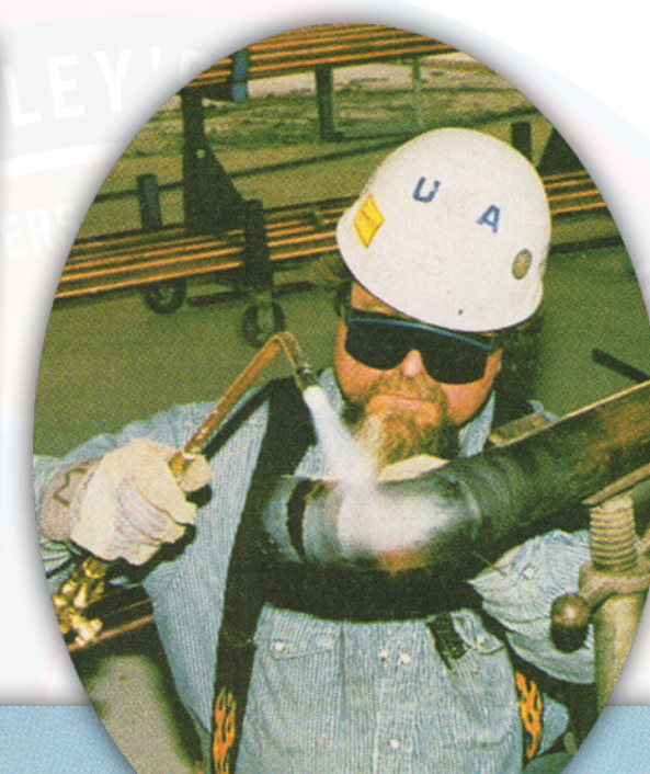
Michael Turnipseed works on construction of the new Valley Children's Hospital in 1997.
