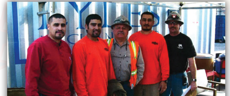
Local 246 members working on the renovation of the B.F. Sisk Courthouse in Fresno in 2010. Pictured left to right: Robert Topete (General Foreman of the job and current Local 246 Business Manager), Marcelo Mercado, Sal Carmona, Frank Flores (current Exam Board Officer), and Danny Wright (previous Local 246 Business Manager).
