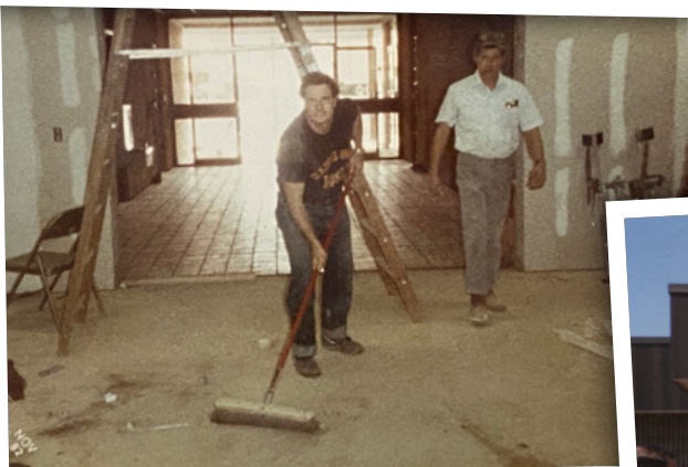
Local 252 constructed and moved into its current Union Hall at 2980 Southampton Road in Northeast Philadelphia in 1982 after breaking ground for the facility on June 4 of that year and hosting an open house and dedication – complete with a toast to the new building – on November 13.
