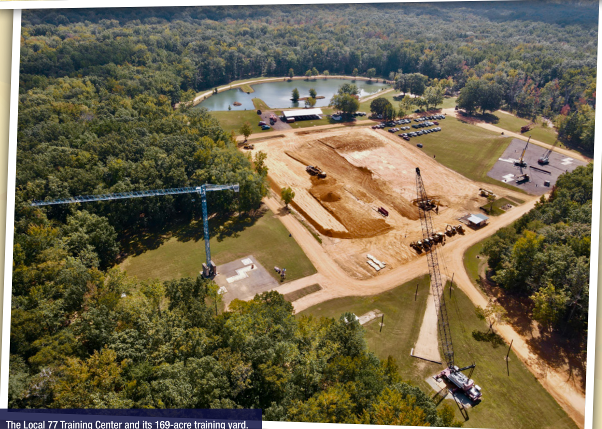
The Local 77 Training Center and its 169-acre training yard.
