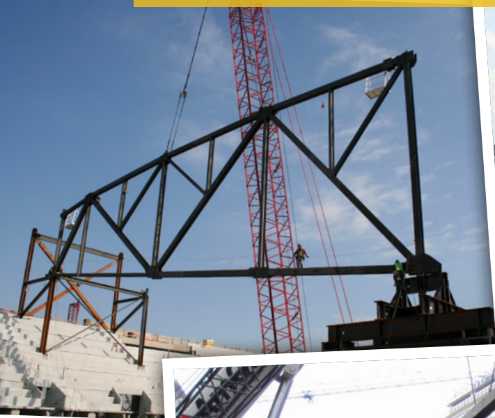
Construction of the KFC Yum! Center indoor arena in downtown Louisville with Local 70 members in 2008 and 2009. (Images compliments of Hillsdale Fabricators.)
