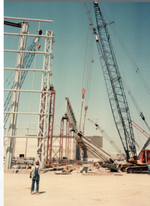
Union ironworkers work on a project at the Dallas-Fort Worth International Airport in 1988.
