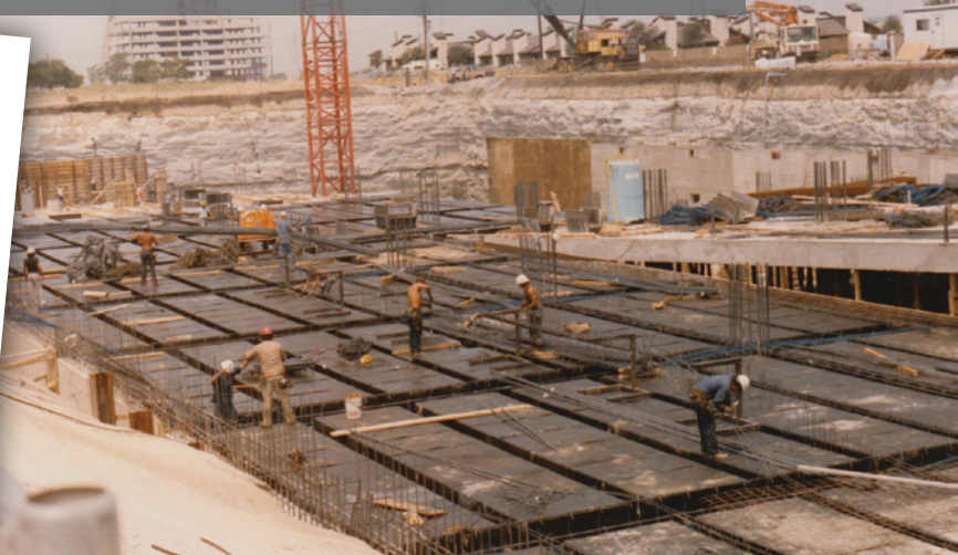
Union ironworkers build the 11-story Stone Tower office building on Noel Road in Dallas in 1984.
